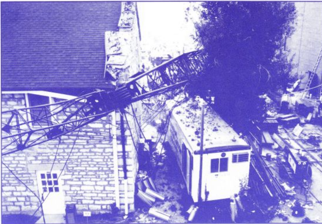
Aug. 18, 1989: The boom of a 70-ton crane collapsed during construction of the E-wing addition. No one was hurt and damage was minor.
