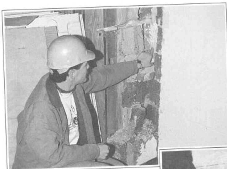
Oscar Revere, construction superintendent, indicates where the limestone lithographic stones remain cemented in the north wall of Erskine Hall, future site of the new entrance way.
