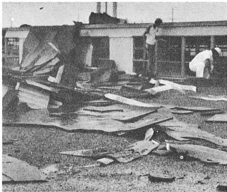
TEN YEARS AGO... Estimators survey damage to the motor-pool building at South Annex caused by a twister.
