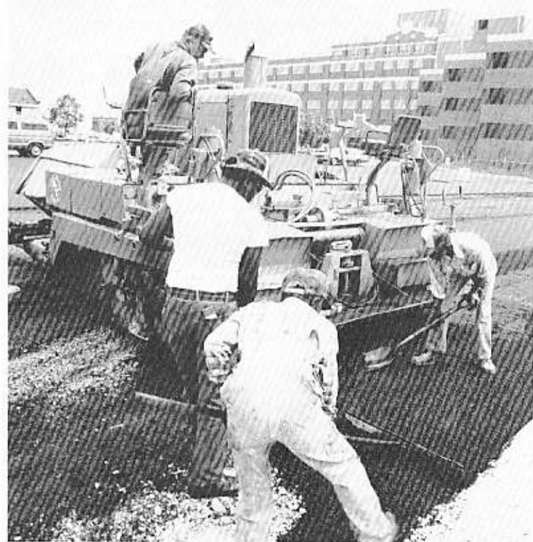
Contractors lay asphalt on the parking lot north of Building 12. Building 36 and E Wing appear in the background. (Photo by Jim Stepanik)
