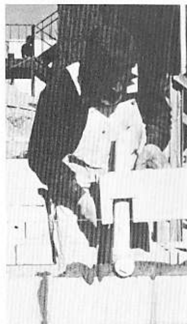
Rich Distler places a concrete block over a plumbing vent during construction work by his church in Mexico.
