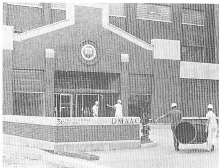
STEPPING FORWARD —Construction workers try out the new main entrance to the Aerospace Center a few weeks before its opening during a ceremony attended by some 2,000 employees and retirees. Dedication of the new entrance and lobby culminated completion of the Building 36 "E" Wing construction project, representing a major step forward in the effort to modernize Aerospace Center facilities.
