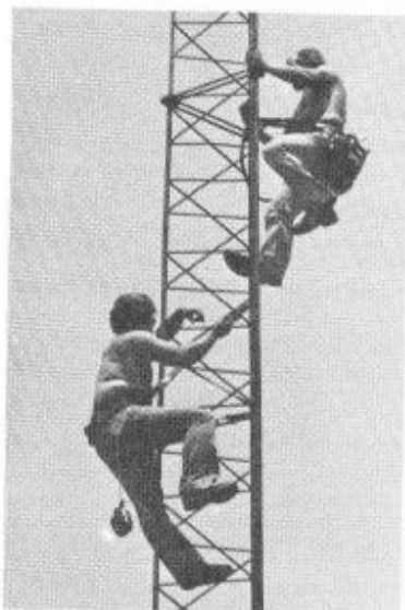
Contractors who had to work outside on the antenna atop of Bldg. 36 coped with the heat by shedding their shirts and carrying canteens of water.
