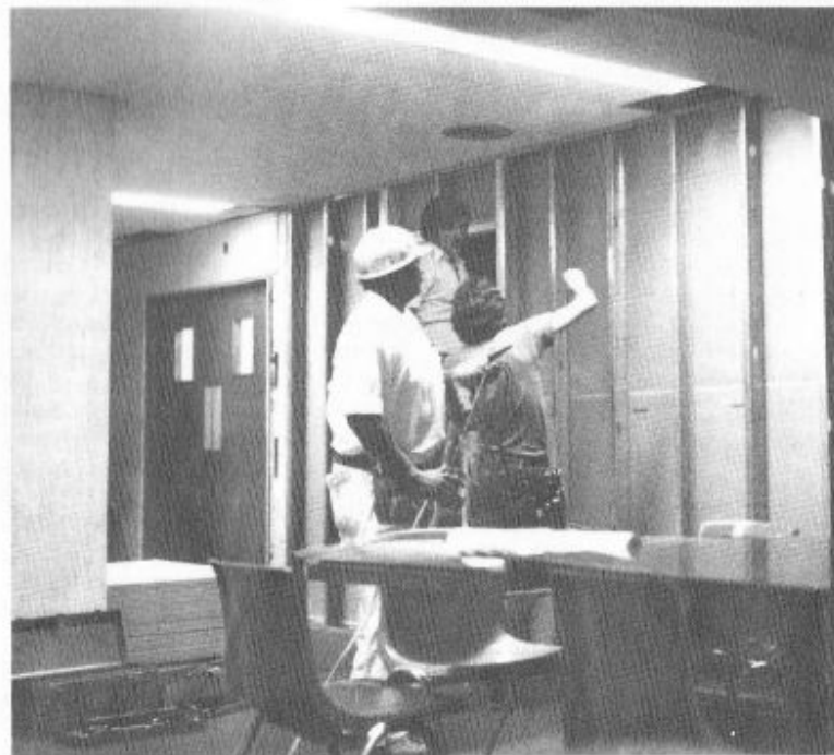
Renovations currently underway at the 2nd Street Dining Hall are funded by the BRC Contingency Reserve.
